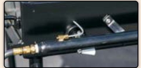
Gas Manifold With Cover Removed
